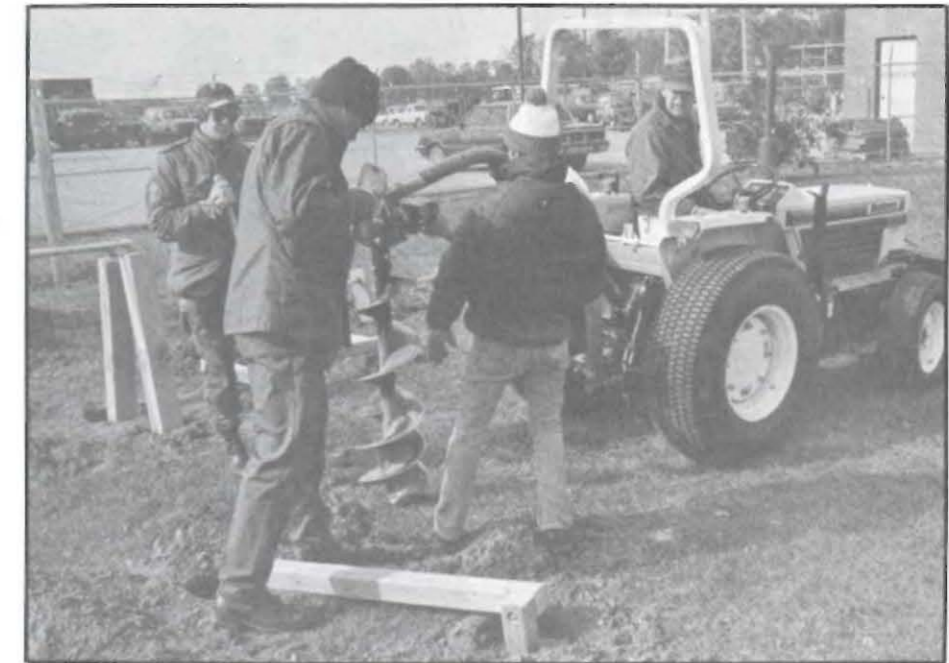
DRILLING -- Installing a post for the base fitness center are (from left) SMSgt. Philip L. Lambers (251st Combat Communications Group), Maj. Eugene W. Brandewie (178th Mission Support Squadron), and TSgt. Stephen M. Thompson and Amn. 1st Class William H. Wendling Jr., both of the 178th Civil Engineering Squadron. (Photos courtesy 178th Tactical Fighter Group Public Affairs Office)
