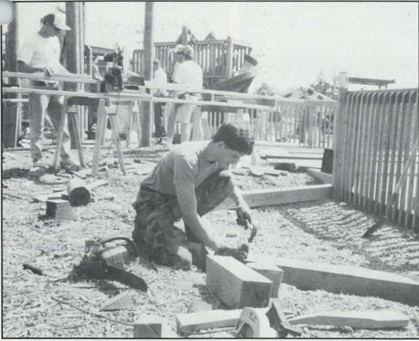
June 13, 1993—After rainy weather slowed the efforts of North Royalton community volunteers building a playground, members of the 112th Eng. Bn. were called in to help. Unit members like Spec. Steve Petroski were happy to lend a hand in the construction of the 15,000 square foot playground.
