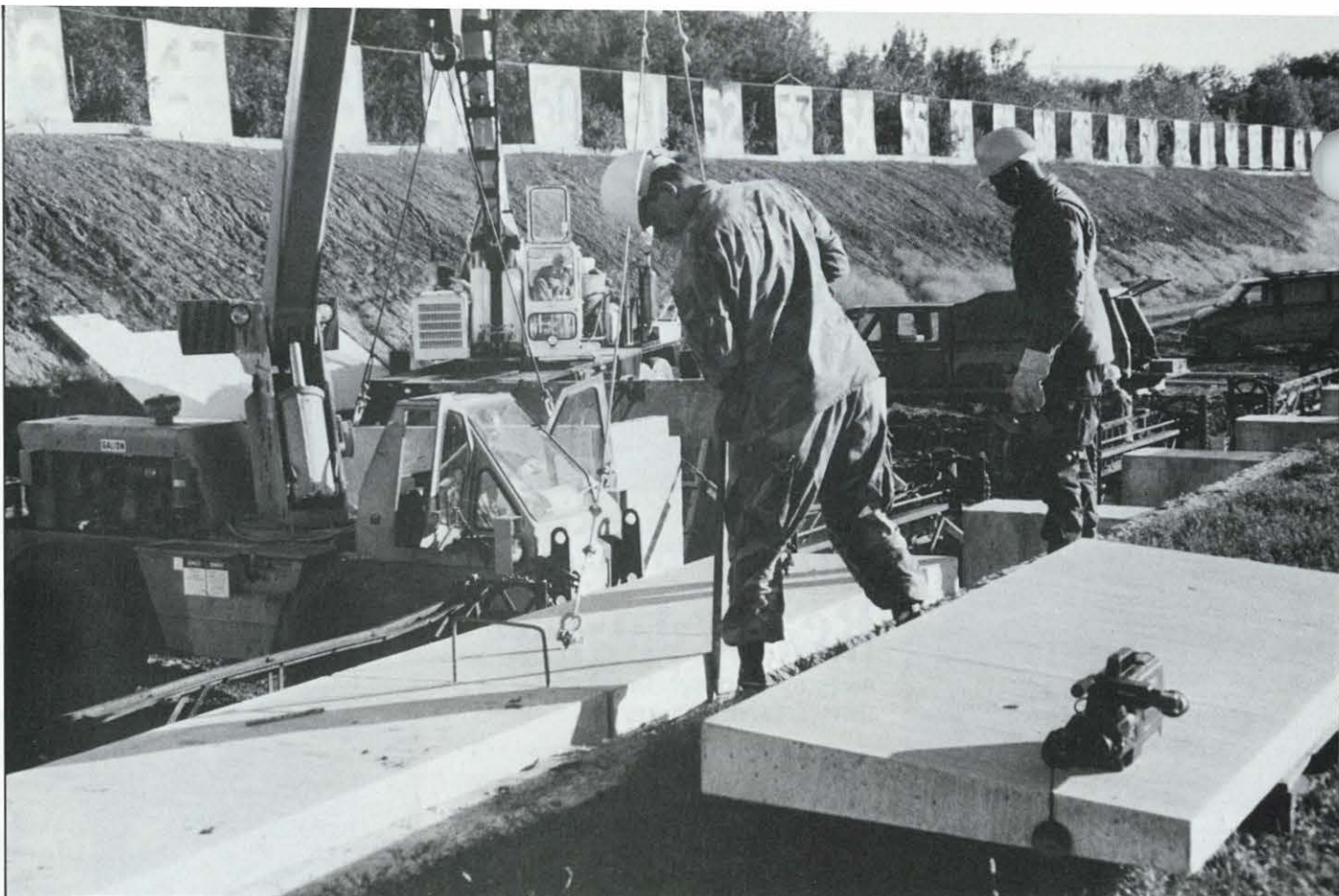
RED HORSE airmen position mantle lids onto wing walls using a Canadian crane. These lids were secured, sealed, then covered with dirt.
