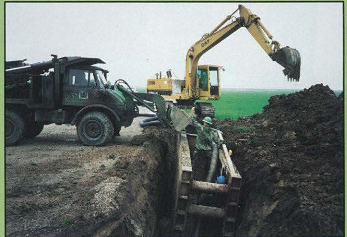
CLOCKWISE FROM LEFT: Aerial view of Young Range after installation of drainage lines. Newly installed ground water lift station pumps drainage into storm water sewer. Members of HHC, 612th Engineer Battalion install drainage tile for the modified record fire range upgrade at Camp Perry.
