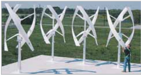
A set of vertical axis wind turbines has recently been installed at Rickenbacker Air National Guard base. (Courtesy photo/ Lt. Col Mike Troxel)
