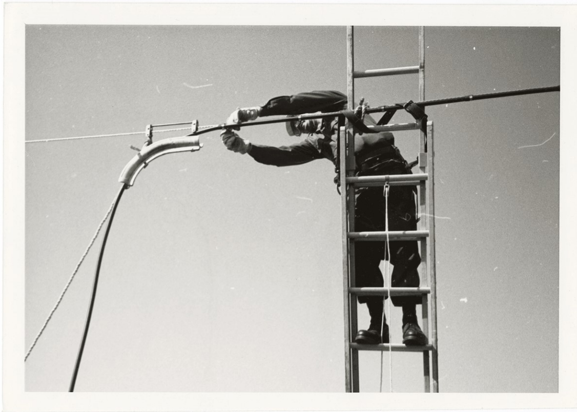
Tech. Sgt. John Lawter straps cable while securely attached to his ladder during the 1984 Air Force Communications Command Engineering Installation Shootout competition.
