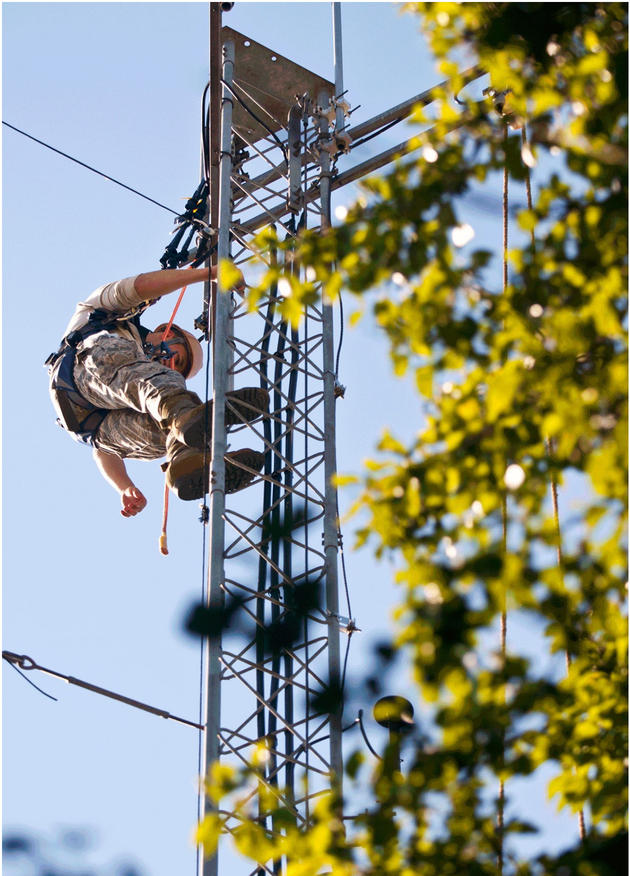
Staff Sgt. Nicholas Norris performs an antenna preventative maintenance inspection perched high on a tower at Rickenbacker Air National Guard Base, July 17, 2014.
