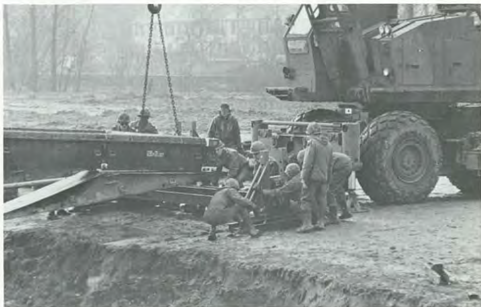
BUILDING A BRIDGE — 1193rd Engineers begin the last phase of work of the medium girder bridge. Use of heavy equipment was necessary to construct the bridge, which is capable of supporting some tracked and most wheeled vehicles. (PHOTO BY Sgt. MARK S. BRACKNEY)
